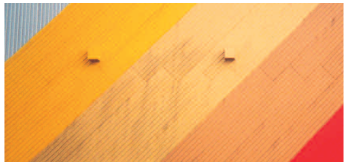
Dirt build up on cladding.
