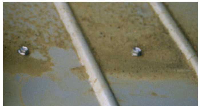
Mould growth on pre-finished steel cladding.
