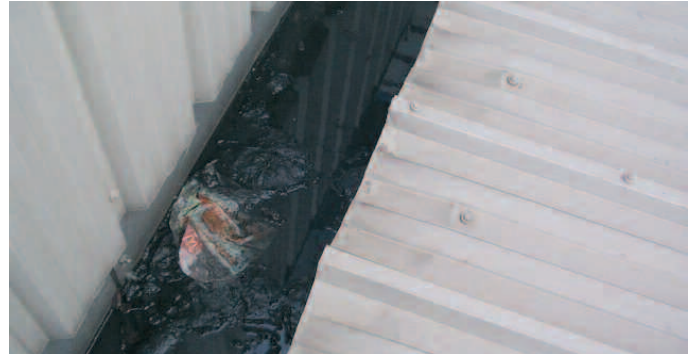
Build up of dirt in a gutter.
